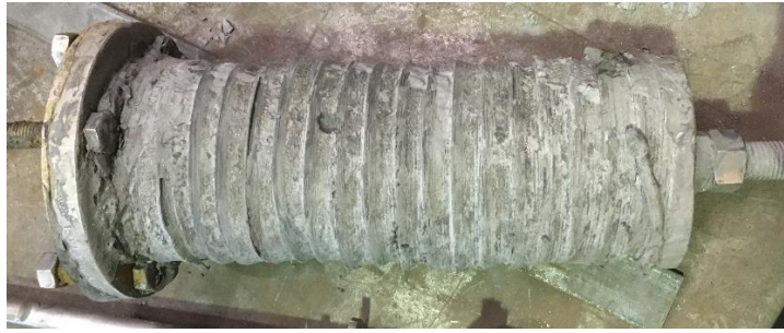
Figure 7 Cylinder gas dispersion system after approx. one year of operation
